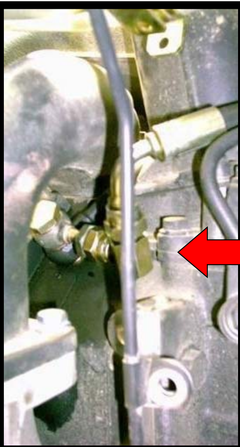
Filter IN (Engine OUT)
