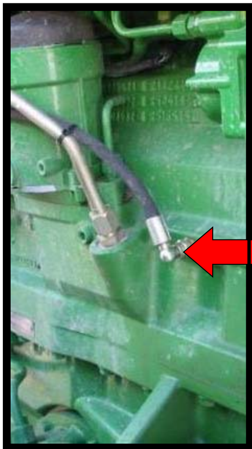
Filter IN (Engine OUT)
